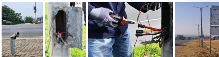
Images: Vandalised streetlights (pre-own-instance investigation) and City Power technical team onsite
