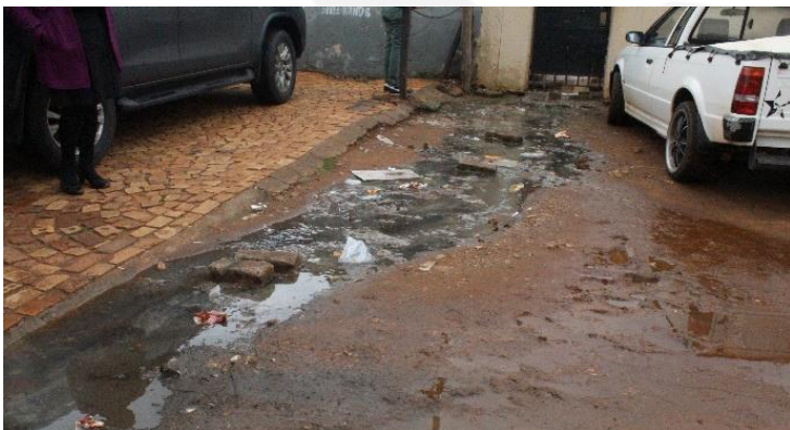
One of the many affected residential homes in Ward 13, Protea South, Soweto
